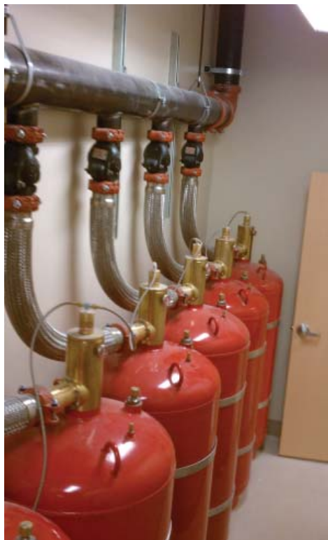
SEVO 1230-500 psi system installed. Photo Courtesy of Phoenix Children's Hospital.
